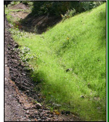
Grass grows a few weeks after hydroseeding a steep road bank in Benson.
