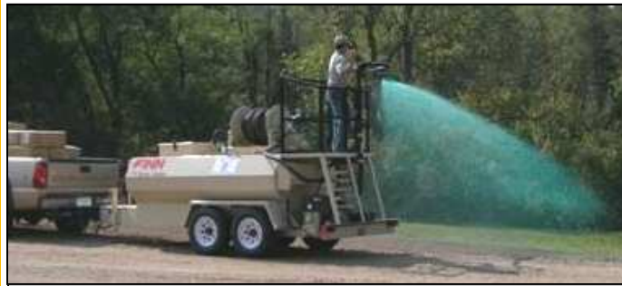
Material is sprayed onto bare soil from the top of the Hydroseeder to prevent erosion.
